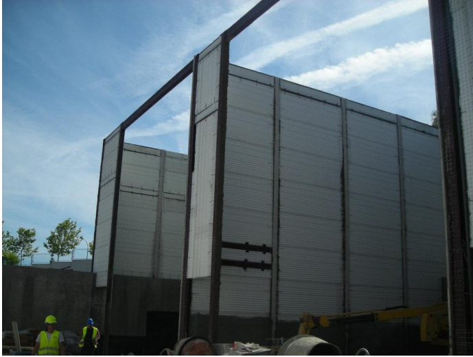
First Iberdrola energy substation built with Baupanel in Madrid, completed August 2012
